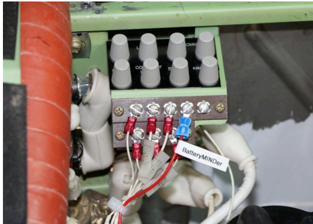
Charger harness wired to battery bus.
